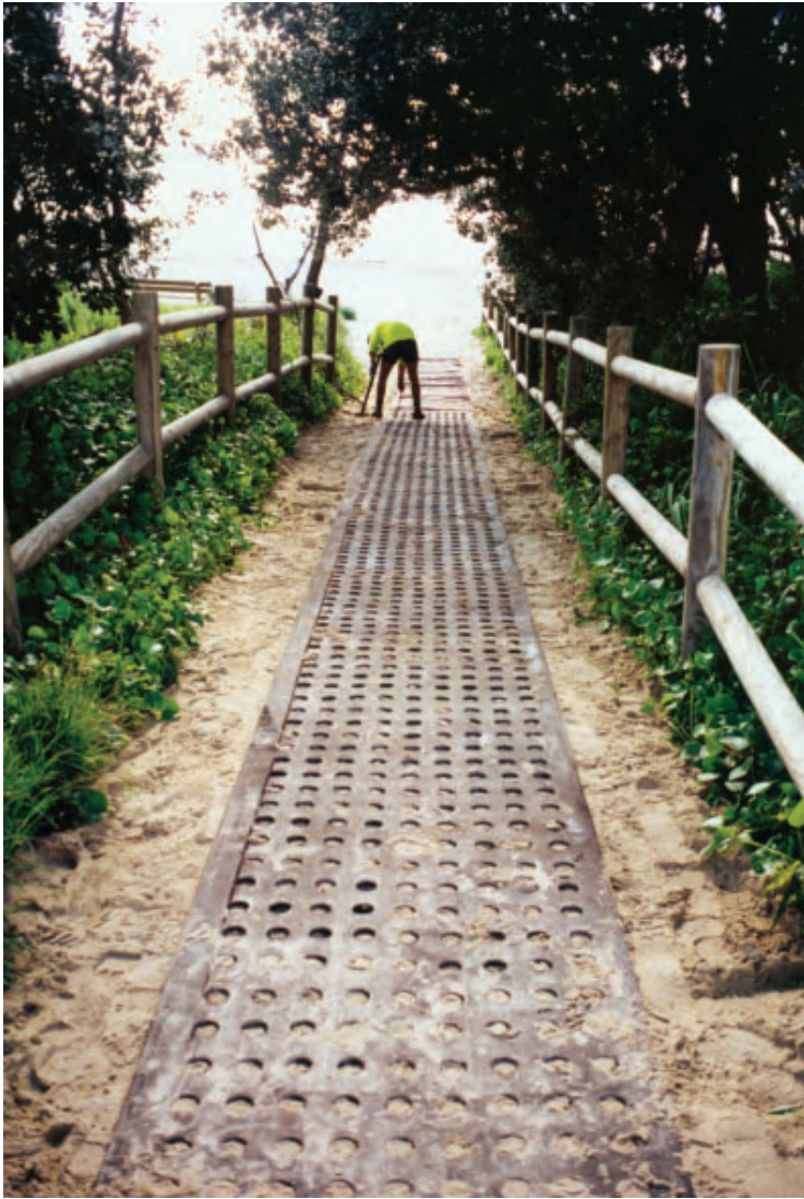
Photo #2. Holeybelt walkway installed by Coastcare NSW provides an attractive and softer alternative to board and chain.
